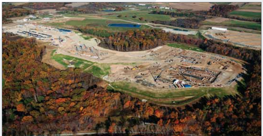
Carroll County Natural Gas Fired Power Plant (Photo courtesy of Mike Sieber/Pipeline Connections)
